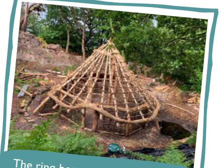
The ring beams making a ladder up the rafters, ready for the thatch roof to be added.
