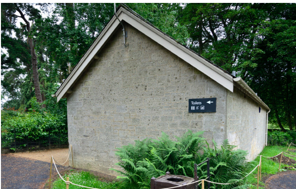
This is the toilet block, where you can stop before you check in.
