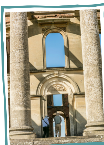
Two of the columns on the south portico at Witley Court and Gardens.
