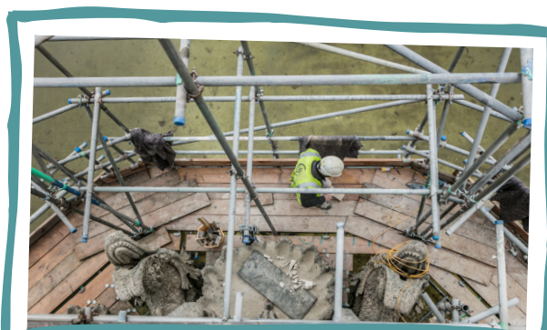
A view from above looking down on the scaffolding that was used during the restoration of the Perseus and Andromeda fountain. Scaffolding is constructed from metal poles and wooden boards to create platforms that are high enough to access all of the fountain.
