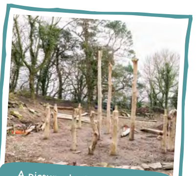
A picture, looking south, of Beeston's roundhouse at this stage of its construction.
