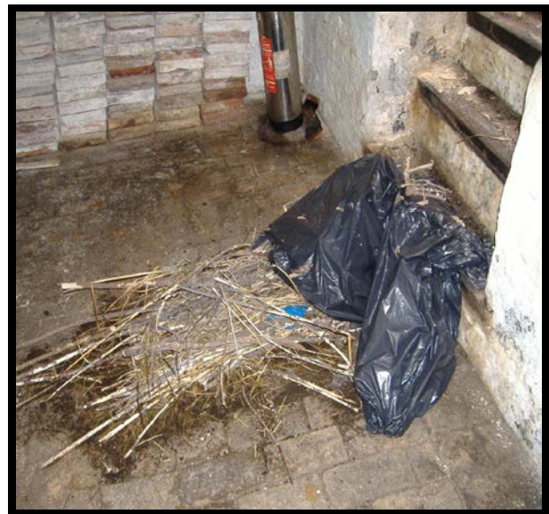
Waste and bin liners in cellar.
