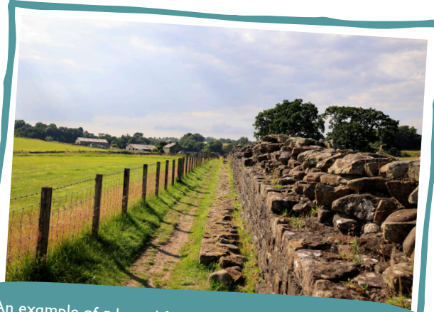
An example of a broad foundation with a narrower wall built on top at Willowford Wall, Turrets and Bridge.
