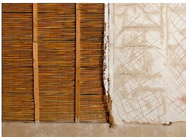
The walls have been left part-finished to display different Roman building techniques.
