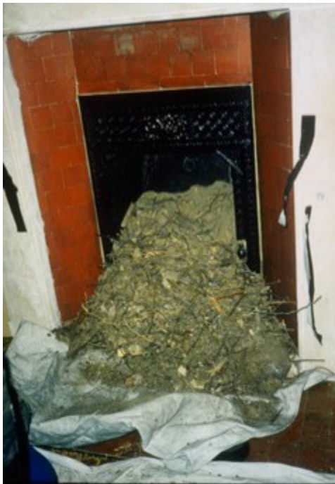
Fig. 3: Fireplace clean in the Duke of Wellington's Room, Walmer Castle, Kent, UK.
