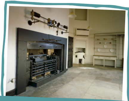
The cooking range in the old kitchen, one of the biggest rooms in the service wing at Kenwood.
