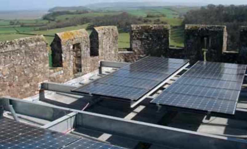
National Trust's photovoltaic cells on the roof of Dunster Castle, Somerset.
