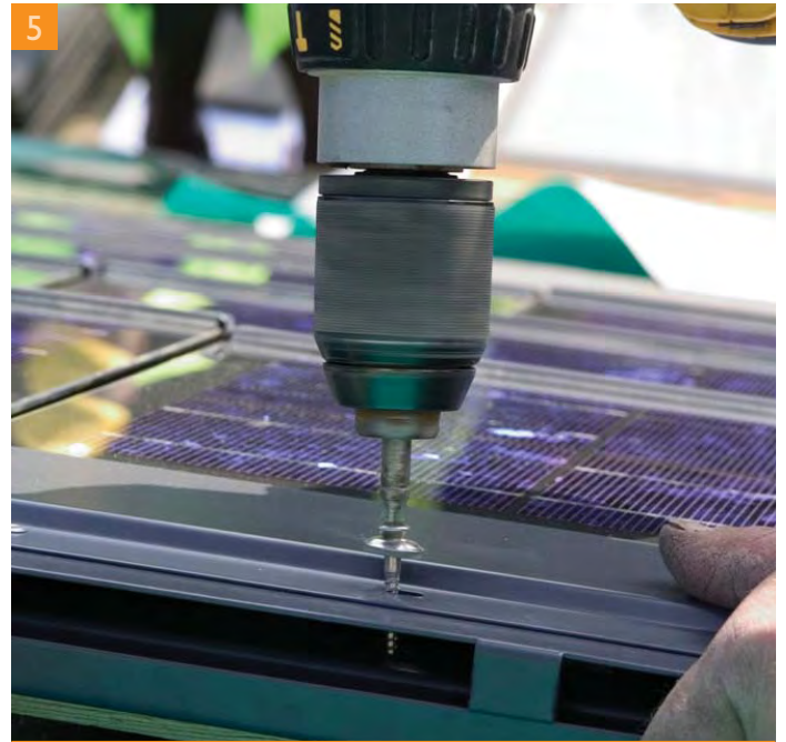
PV roof tile being drilled to timber roof batten. (Photograph courtesy of Solar Century)
