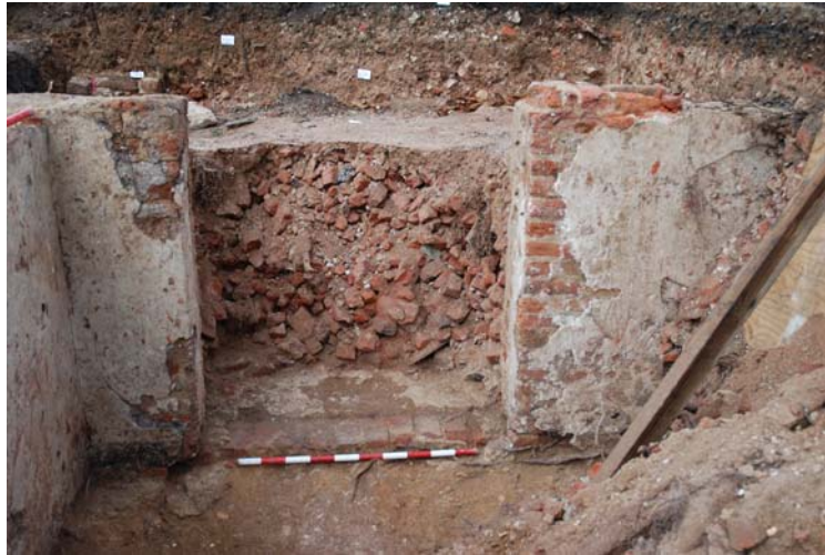
Photograph showing a door opening in the rubble-filled basement (1m scale is laid on the mortar flooring surface)
