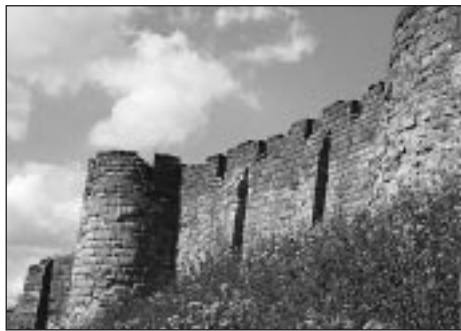
Buttresses along the curtain wall. Ask pupils why they had to be added later. (The castle was known to have needed considerable amount of money spent on it to maintain its defences.)
