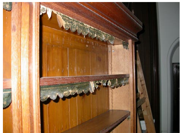
Figure 8. Damaged dust falls at Penrhyn Castle (National Trust), demonstrate the extent of cumulative abrasion that occurs between book spine and dust fall when books are removed from and returned to the shelves.
