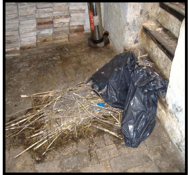
Waste and bin liners in cellar.
