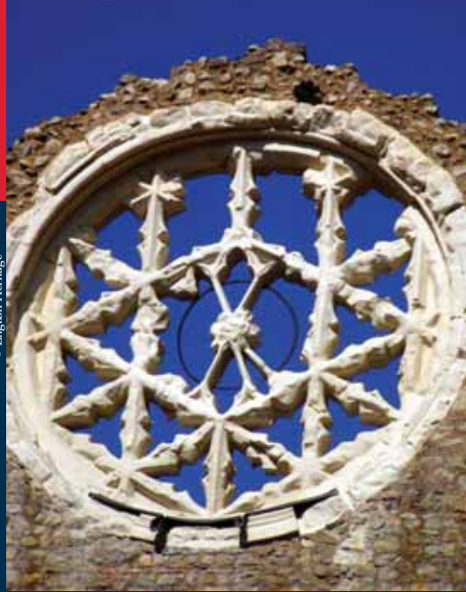
English Heritage carried out major masonry repairs to the standing remains of Winchester Palace
