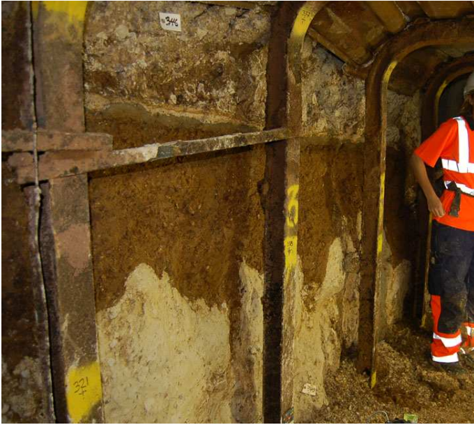
The old ground surface is clearly visible as a thin seam in the side of the tunnel (above).
