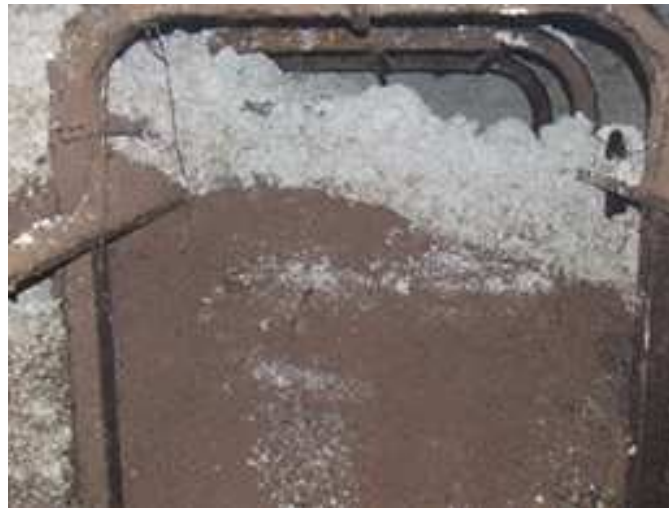
The chalk above the reddy brown fill in the picture above is 1970s collapse caused by the lack of roadstone fill beyond this point.
