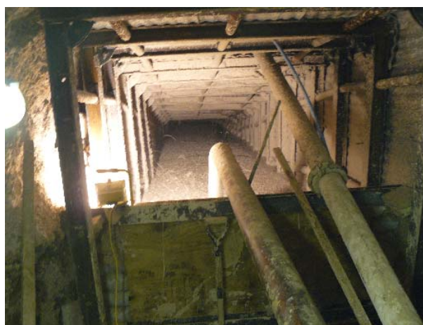
Figure 2: A typical stop-end wall constructed in the tunnel to compartmentalise the paste backfilling
