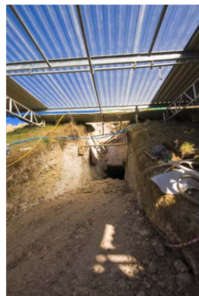
Figure 3: the tunnel area following removal of the door, lintel and initial tunnel portal area
